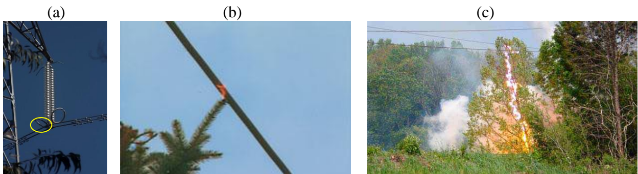
Figure 3. Images showing an example of electric poles, electric discharge, and fire ignition. (a) Detail of a cable joint/coupling; (b) example of air ionization caused by the proximity of a tree branch; (c) fire ignition caused by an electric discharge.
